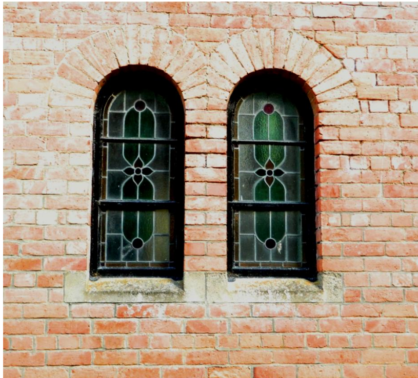
Windows (exterior view), St Luke's, Ardee Mental Hospital (Photographed by L. Butterly, 2012)
